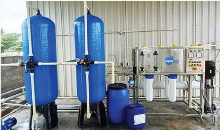
RO water plants (250 LPH capacity) in Gadag and Raichur
